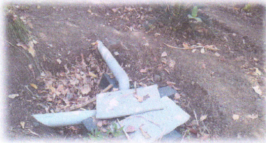
Rain water harvesting Recharging facility
